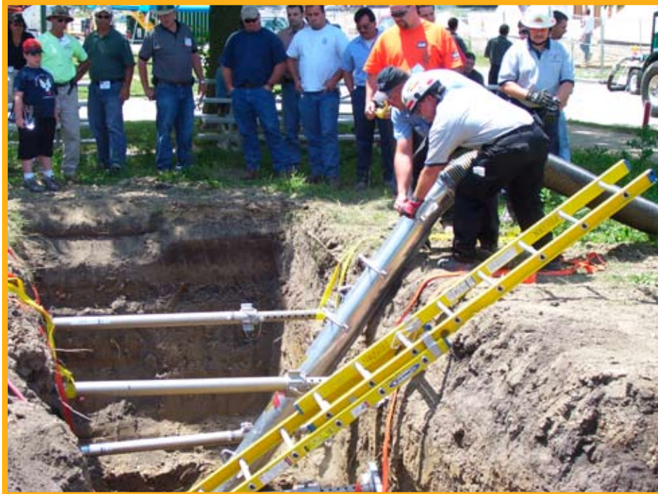
Digging a trench should be considered a very dangerous task. The best way to prevent an accident is good preplanning.
