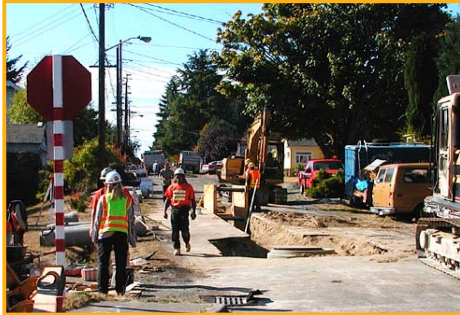
Protective systems are required in all trenches deeper than four feet and where potential for cave-in exists.
