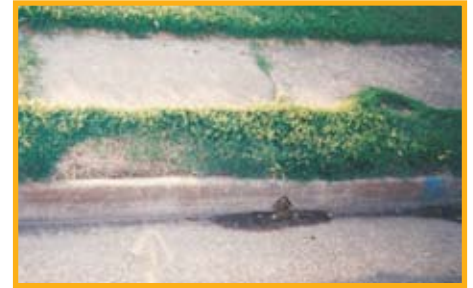
A burn mark located at curb beyond yellow arrow.
